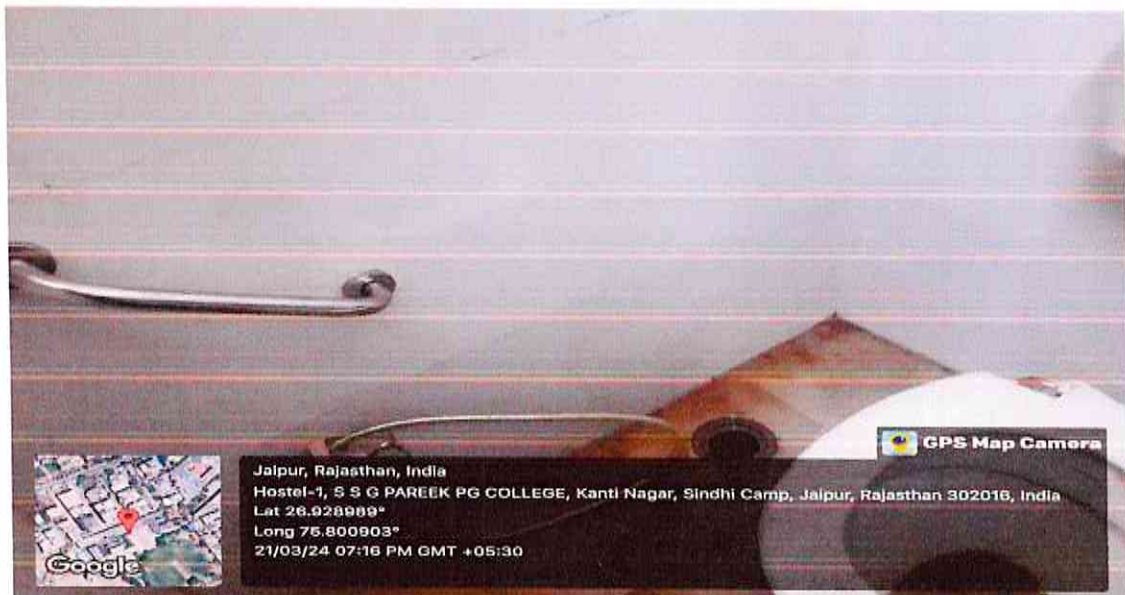
Divyang Toilet in Main Block
