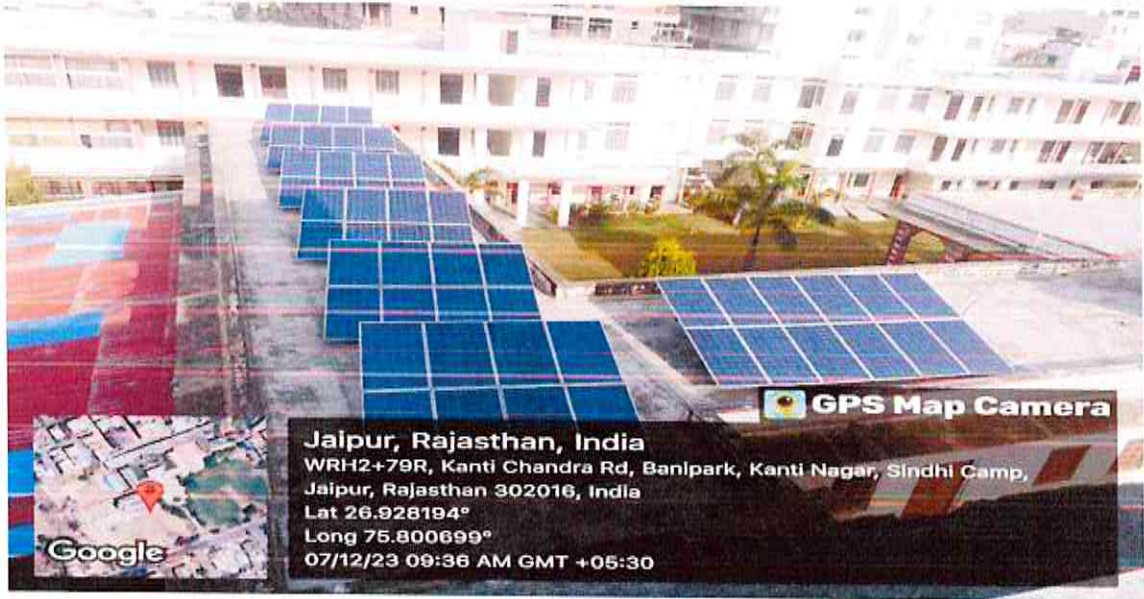
Solar Panel on main Block
